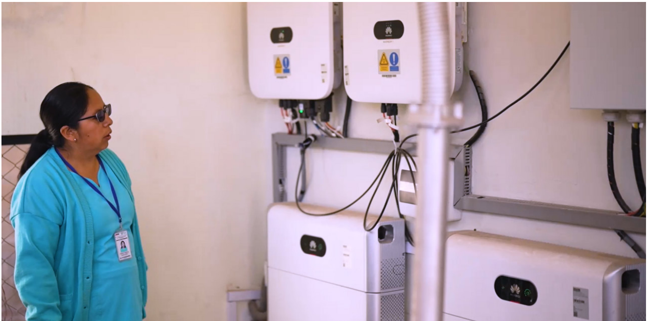
Comprehensive Smart PV+ESS solution for a medical institution in Peru
