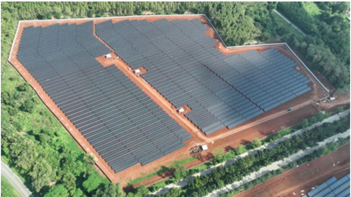
Karawang ground-mounted PV project in Indonesia
